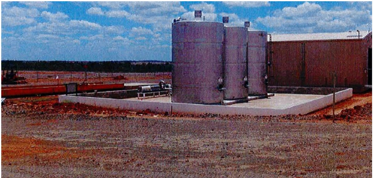
Figure 6: Tanks for Storage of Finished Product – illustration of similar facility
